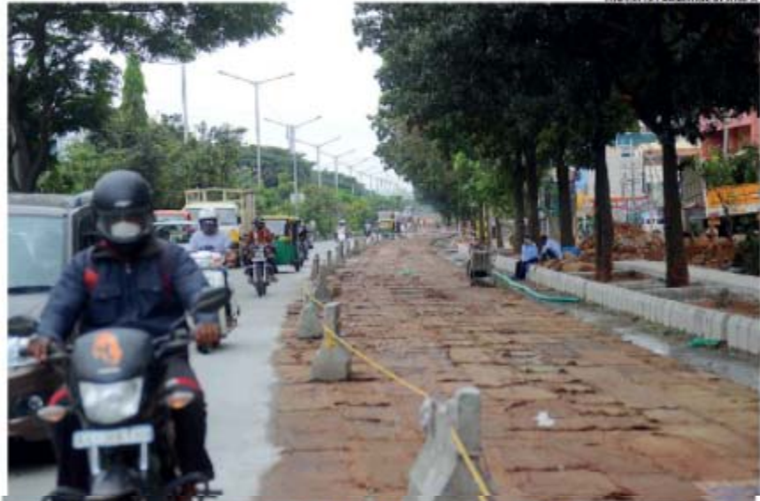
After being stuck for months, white-topping work has begun on Laggere, ORR
